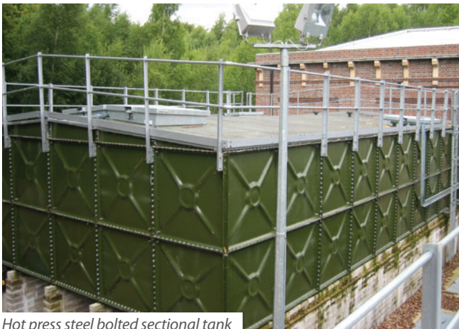
Hot press steel bolted sectional tank
