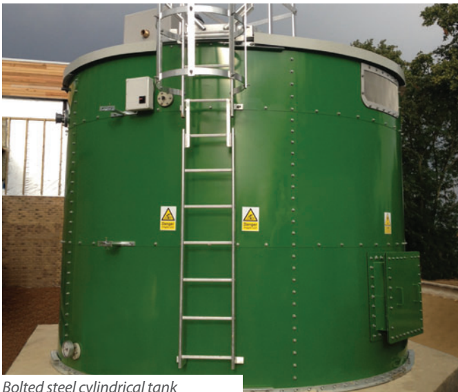
Bolted steel cylindrical tank
